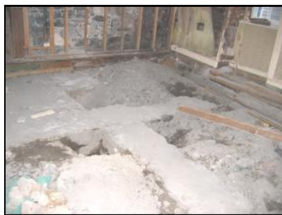
Selective demolition work in summer/autumn 2005 revealed these archaeological vestiges underneath the old kitchen floor
